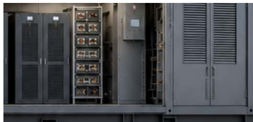
UPS + CONTROLS Critical power and monitoring
