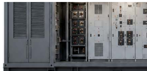
MV / LV SWITCHGEAR Main distribution lineup
